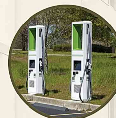
EV CHARGING POINT
